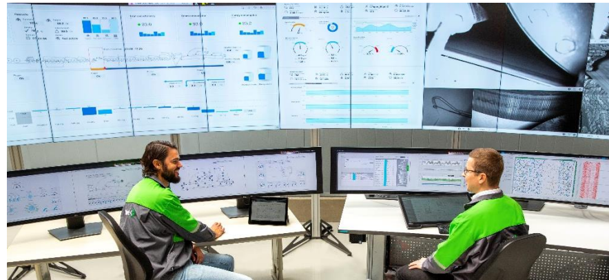
SMALL, MEDIUM & LARGE CENTRALIZED CONTROL ROOMS
